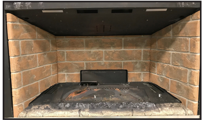
Figure 8 Refractory Kit Installed
