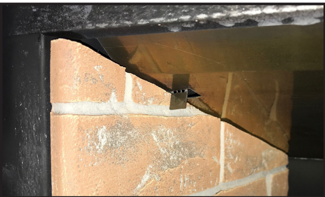
Figure 6 Left Refractory Handbend Tab
